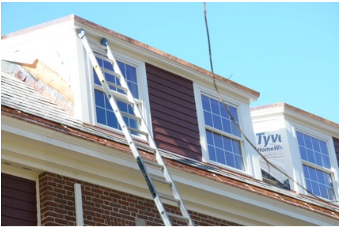
New rear siding, flashing, and the new slate is up on the roof front and back, too.
