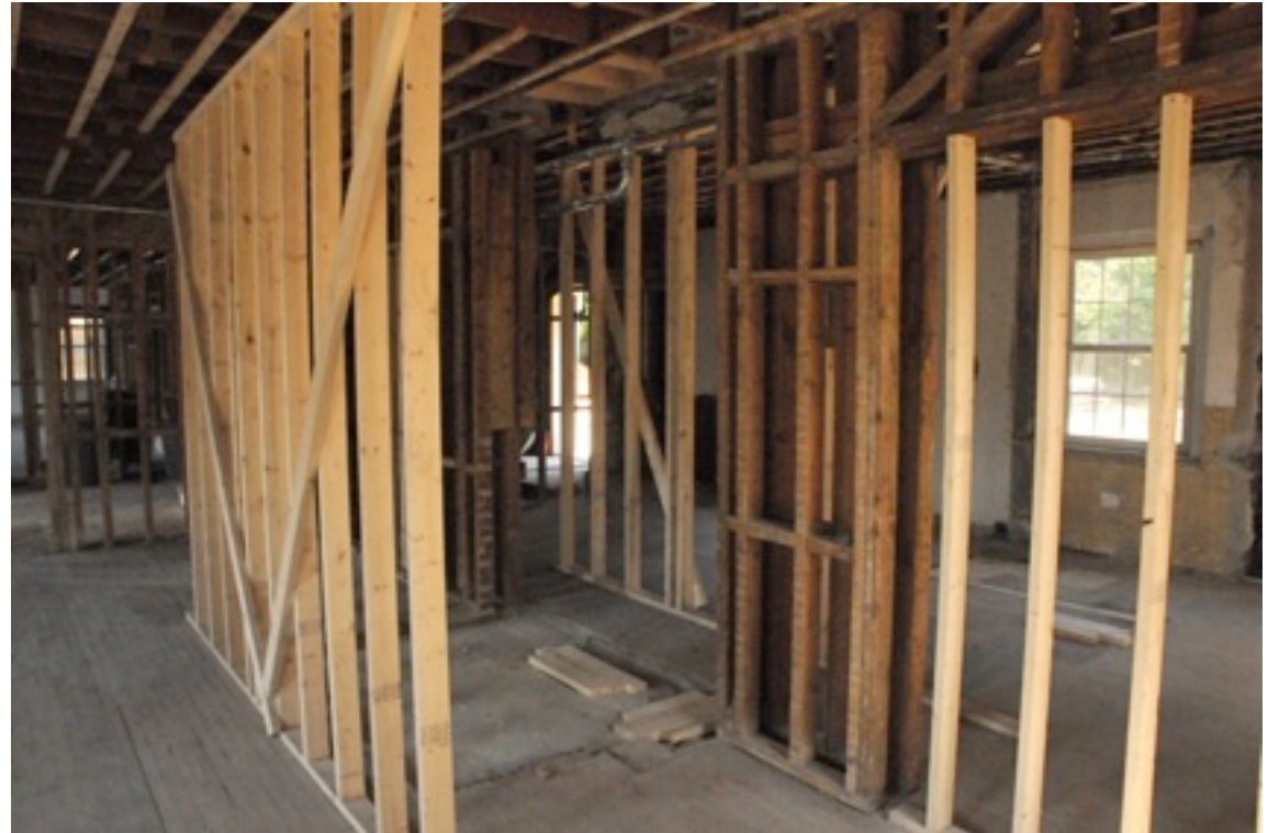
Fire place without the mantel on Aug. 22, 2009 (left) and another side shot on Sept. 1, 2009. Note the framing to the left of the right-hand picture is only for support purposes.
