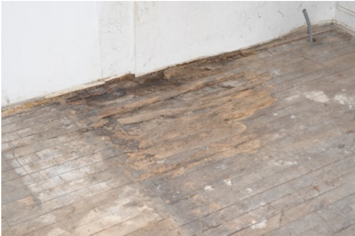
Rotted wood where the sinks were
