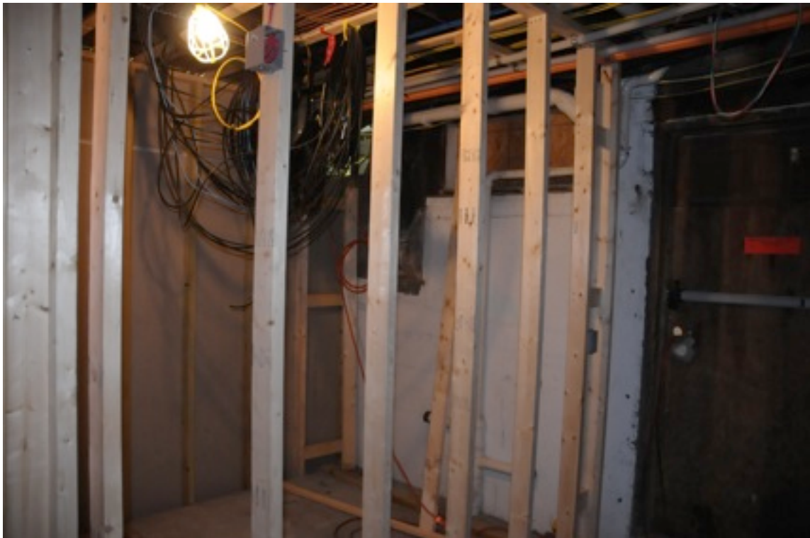
Home to the nerve center of wires for the junction box, and a host of other things. Located downstairs, next to the door to the outside.
