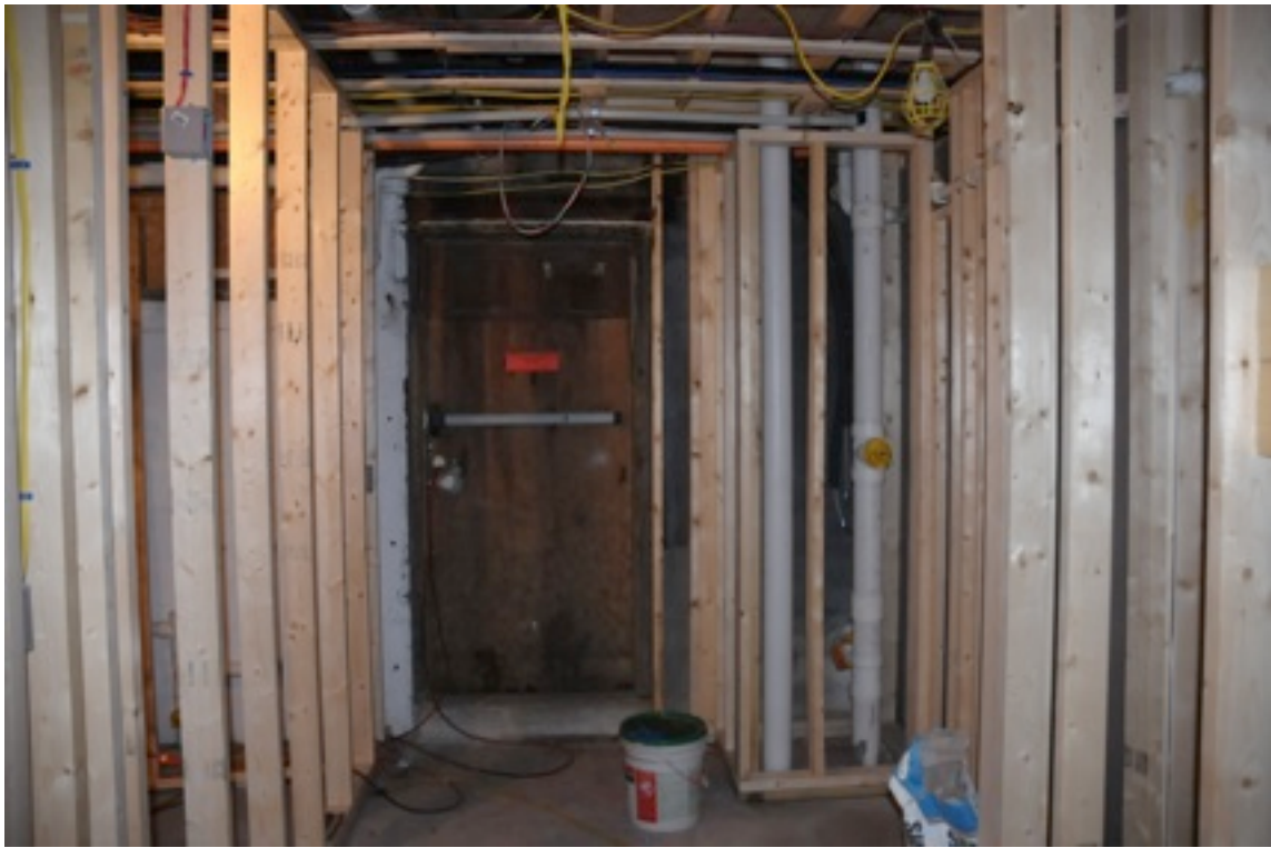
Framing to the outdoor stairway that leads up to the parking lot from the basement
