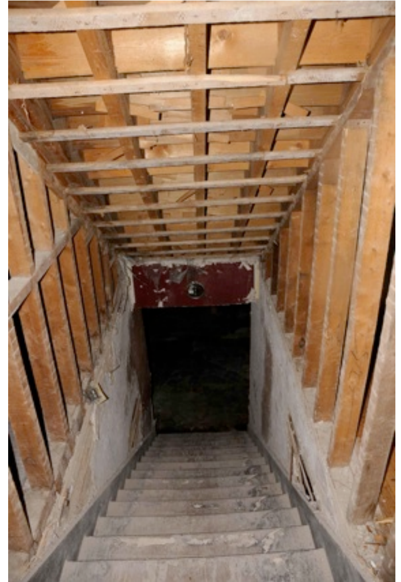
First Floor down into Party Room and the renovated and staircase in the front hallway on Saturday 8-22-09.
