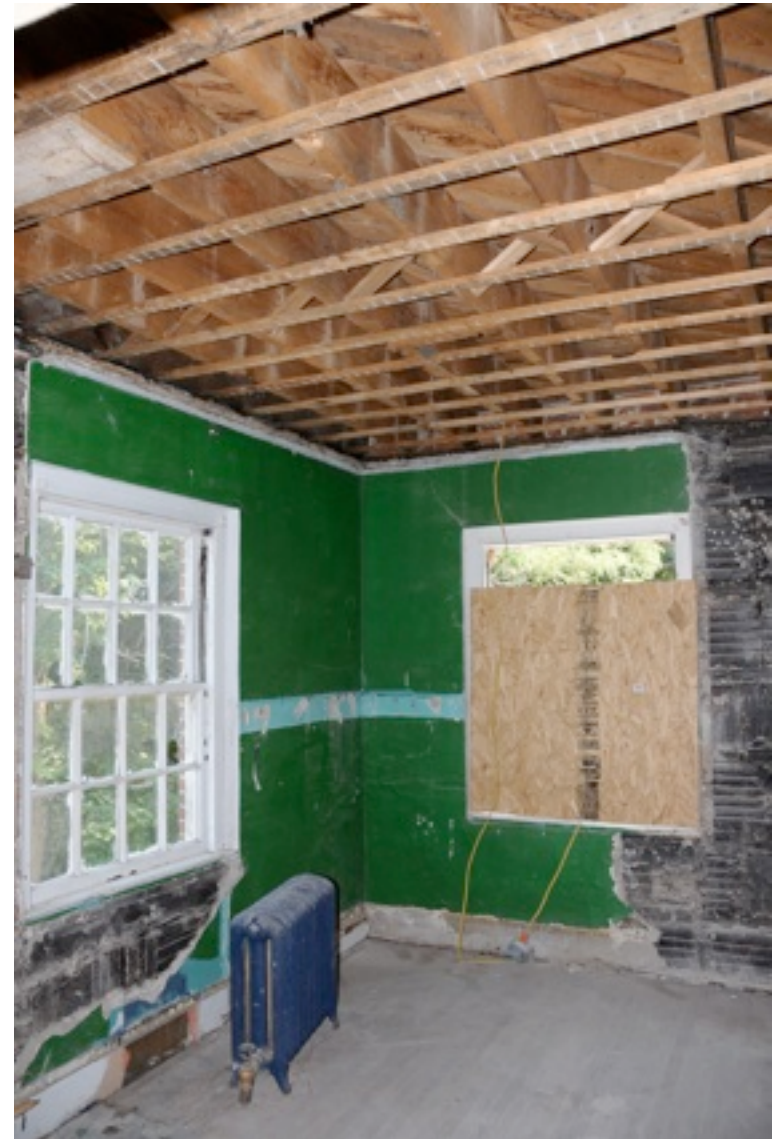
Room that used to have the fire escape access to it on second floor
