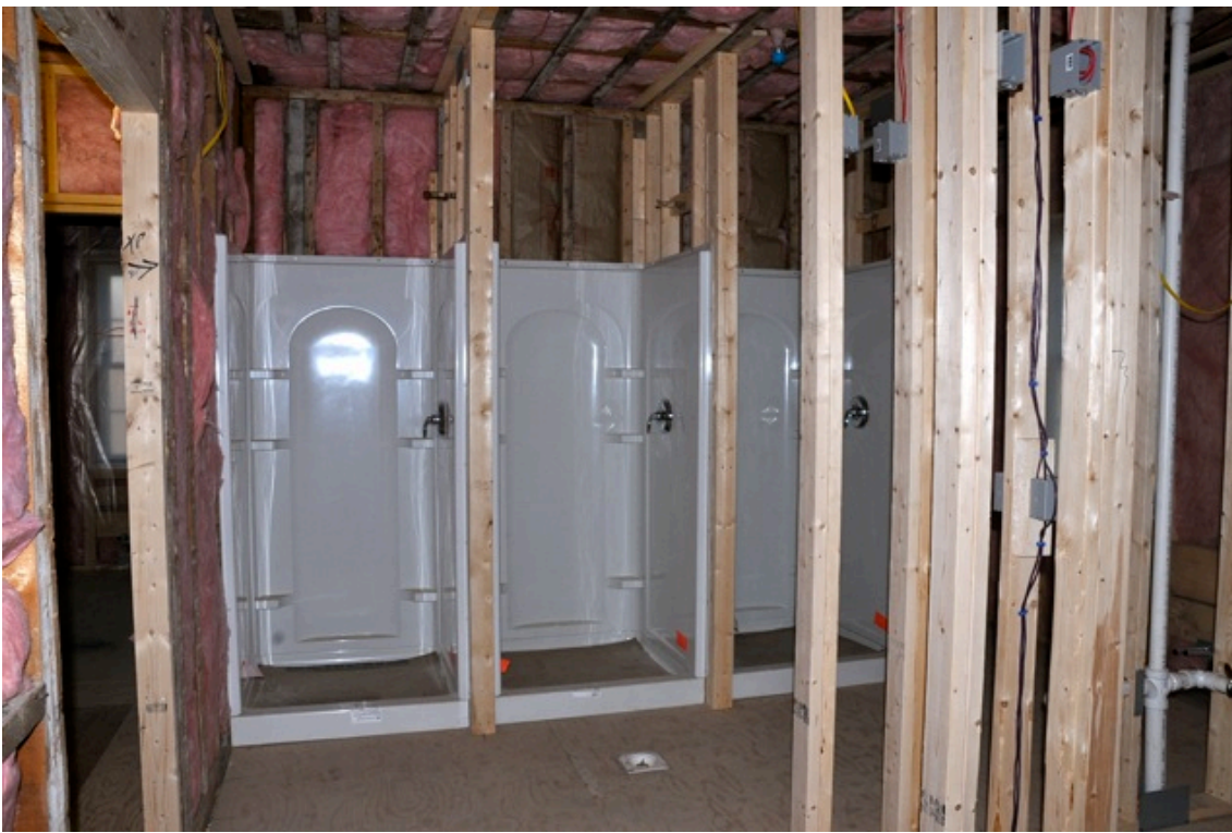
The Second Floor bathroom will have 3 showers and sink setups on the opposite side. It's a great setup once you get to walk around in it.
