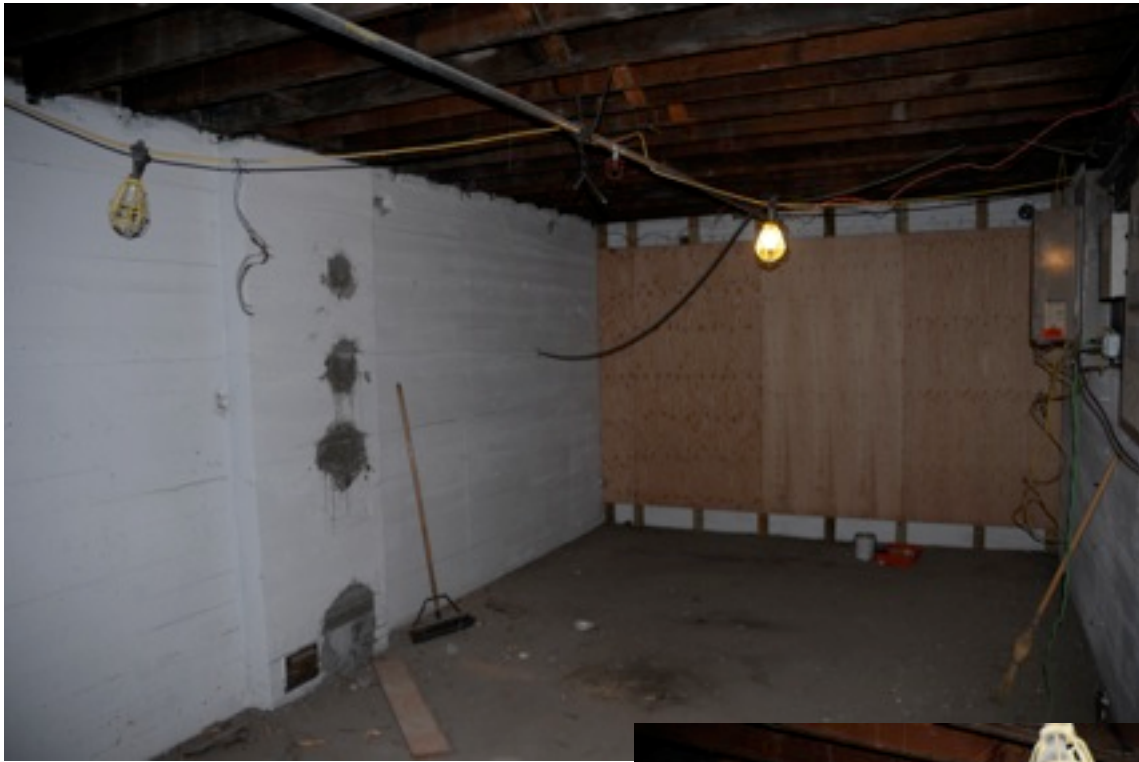
The Cleaned out, cleaned up area of the old Boiler Room down in the basement.
