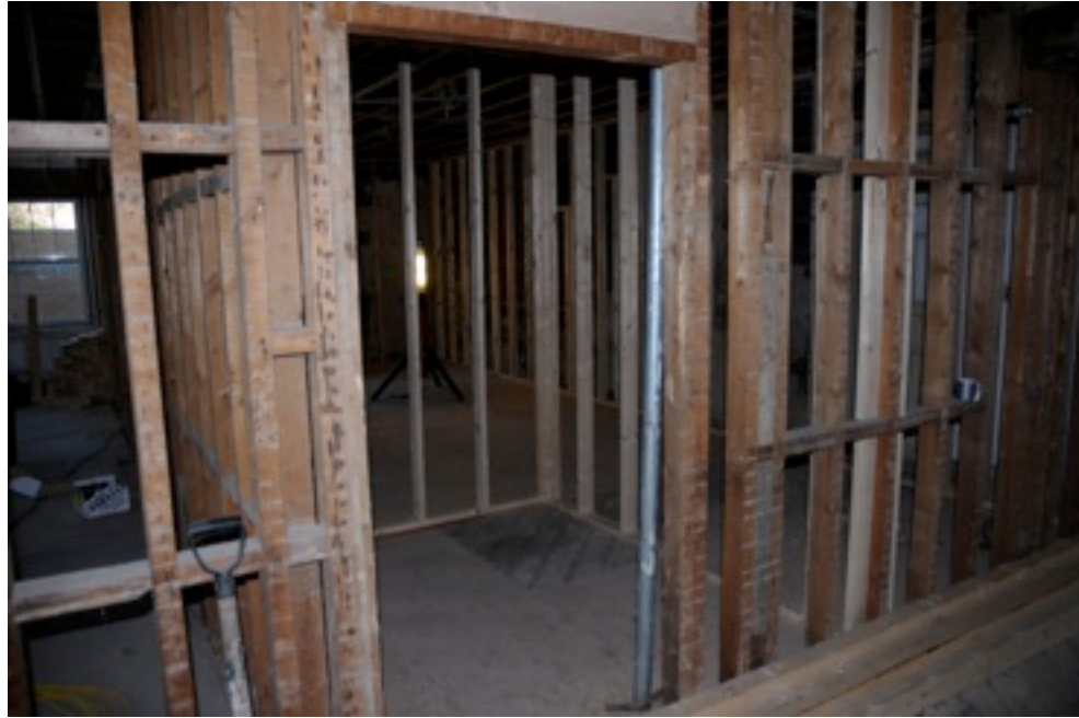
The new women's bathroom that is also wider and now handicapped accessible, still located on the first floor in the main hallway across the main stairwell.
